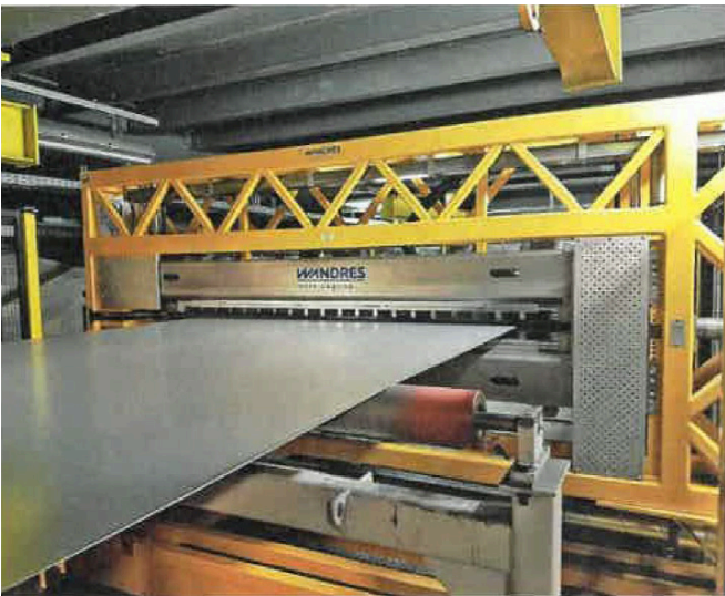
The Cevomat cleans steel strip at a galvanising plant using brush cleaning technology.
